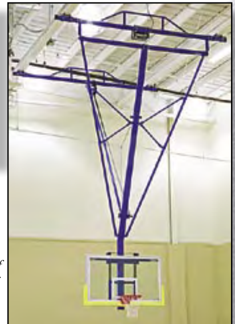
TB-25S-B at Christian Academy of Indiana, New Albany, IN. Architect: MECA Design Group, Greenwood, IN. Photography: Wayne Williams, Indianapolis, IN.
